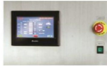
Online monitor performance of washing through test conductivity of water
